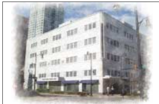
▲ – THE KRESS BUILDING – The 1939 Great Depression-era building is being renovated by the law firm of Wiggins, Childs, Quinn & Pantazis, PC for their new offices.
